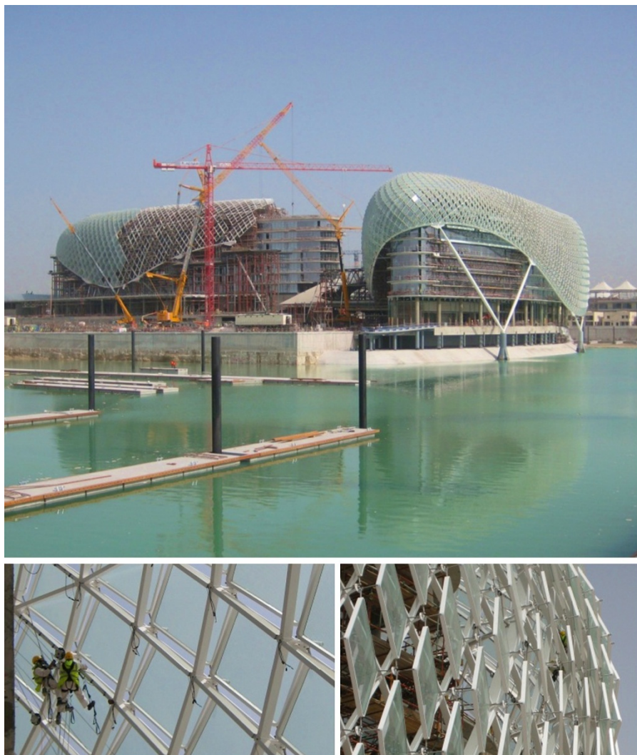
Fig. 4 Yas Island Hotel during construction. At bottom left one can see a detail of the outer skin which exhibits torsion-free nodes (images courtesy Waagner-Biro Stahlbau).
